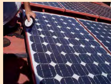
Less obvious fractured glass
