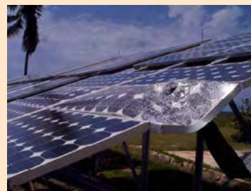
Obvious impact damage
