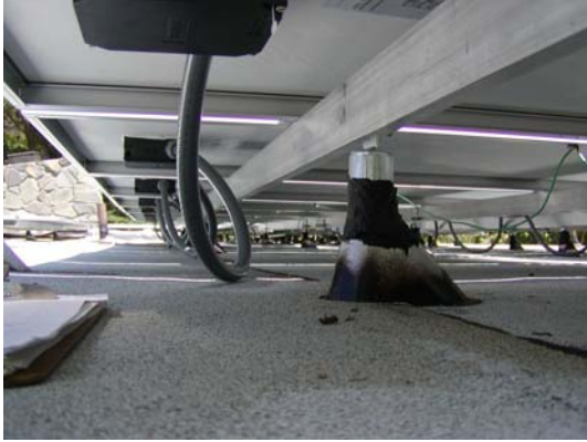
Figure 5 (incorrect) Flex exposed to physical damage
