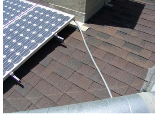
Figure 6 (incorrect) Flex conduit run without support
