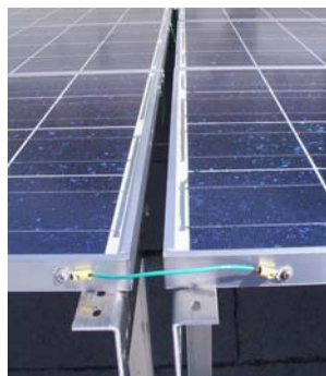
Figure 3 (incorrect) Improper lugs and conduit wire used
