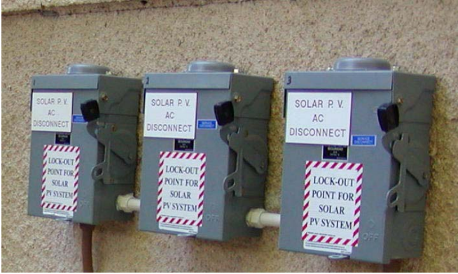
Figure 12 PV System Disconnect Signs
