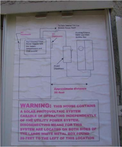
Figure 14 Close-up of sign for emergency personnel
